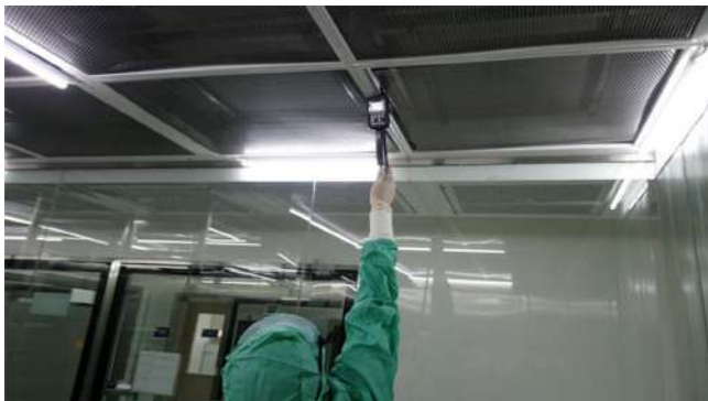
Medical facilities and cleanrooms
