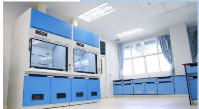
Biosafety cabinets and fume hoods
